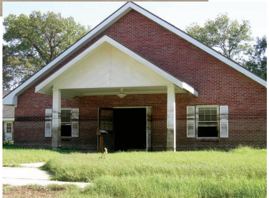
This building in a Kansas community shows the effects of flooding on a site that nobody had seen flood before.
