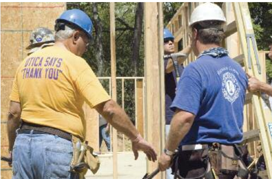
Many of the volunteers—here working on the Howard home on 1st Street—wore t-shirts bearing the names of their hometowns. Many of the volunteers came from communities helped in previous years by New York Says Thank You.
