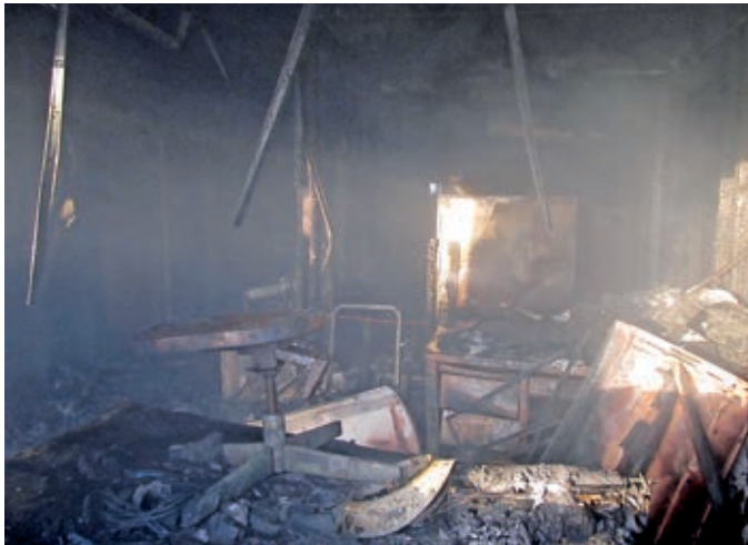
The fire-gutted interior of Rison City Hall the morning after the arsonist struck.
