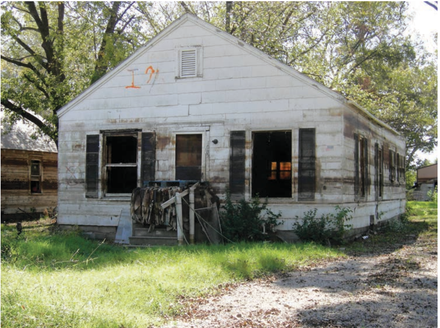
The presence of dilapidated and abandoned housing is emerging as a major issue in many Arkansas cities and is a primary focus of planning efforts.
