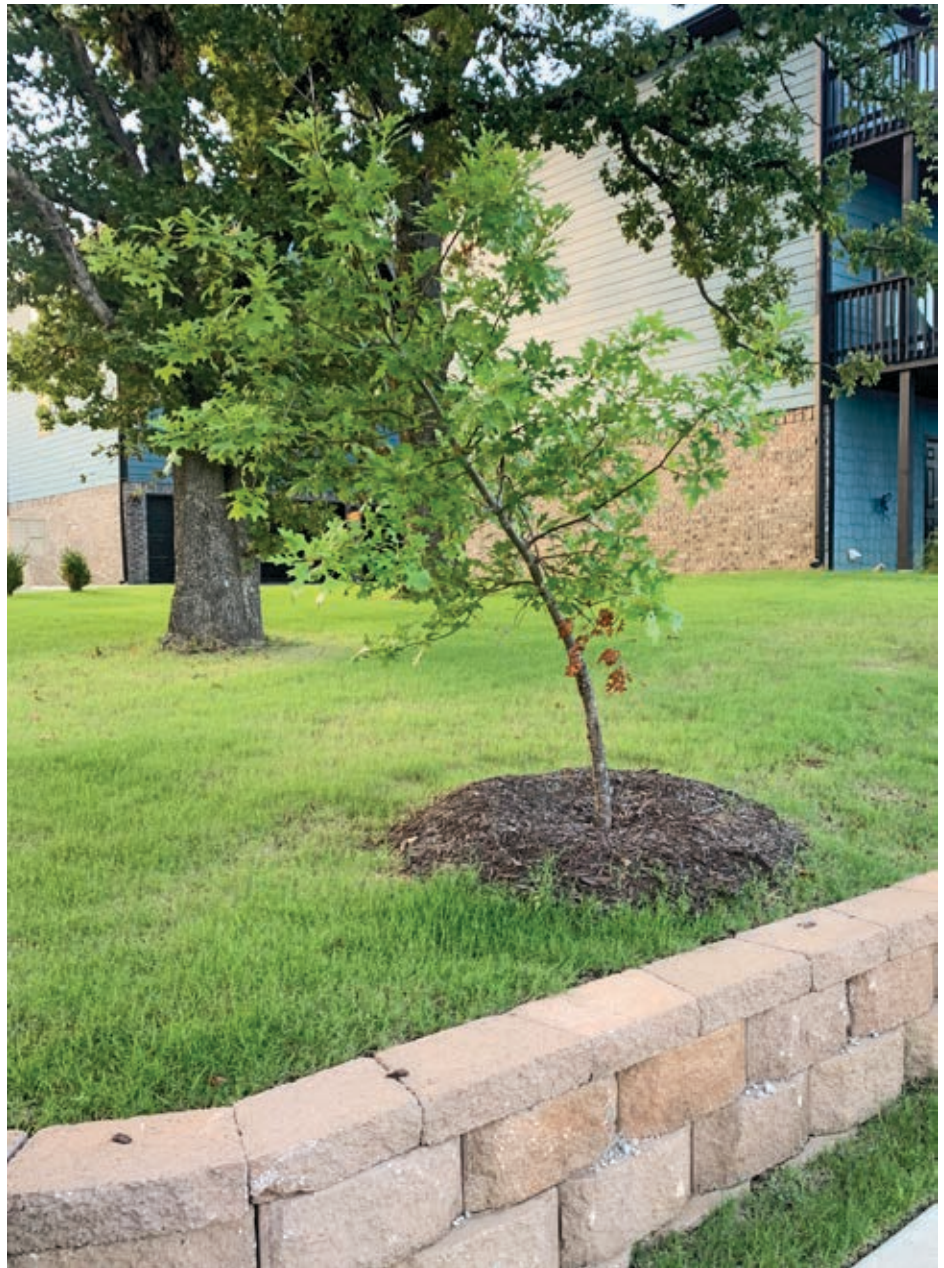
This newly planted oak tree is planted too close to the retaining wall and will eventually cause the wall to fail as the tree grows to maturity.
