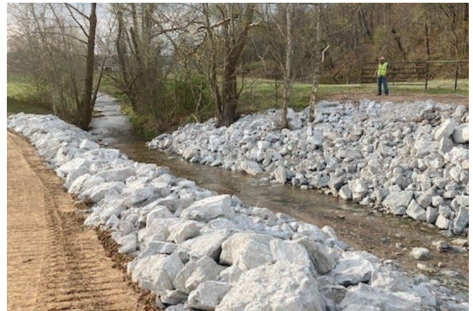
Bank stabilization (above) and elevated bridges at low-water crossings (facing page) are a few examples of projects eligible for mitigation assistance.
