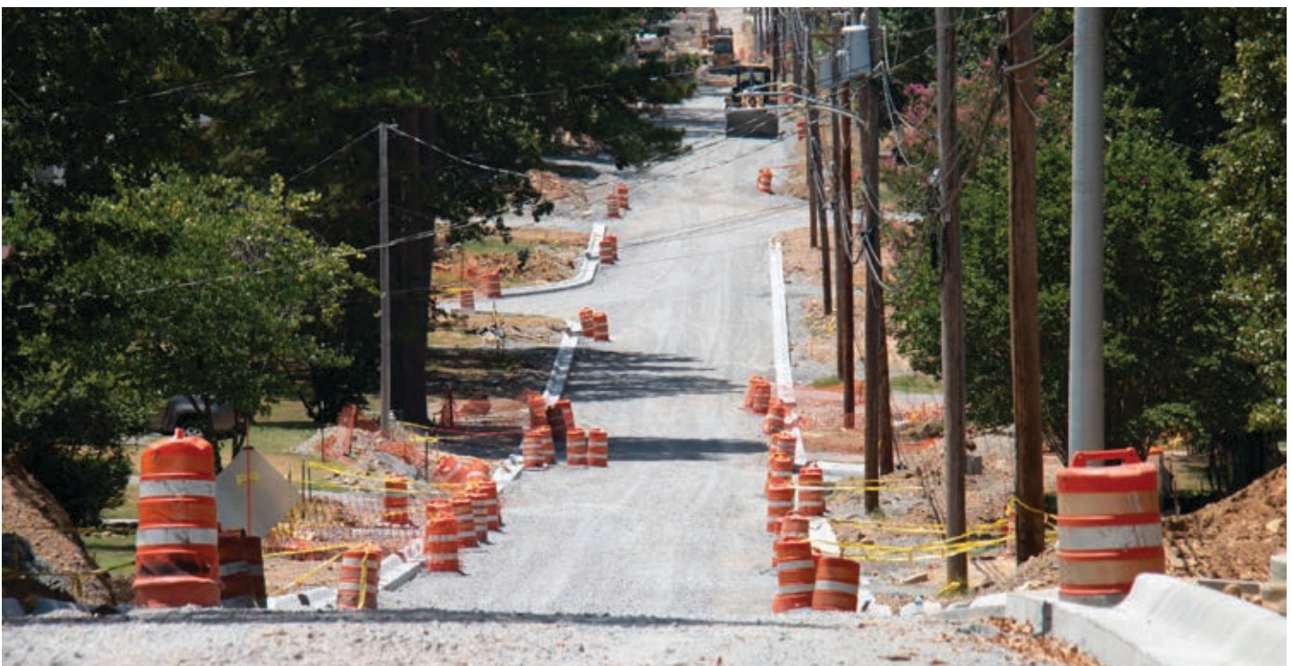
Country Club Drive, the city’s oldest street and a major connector between Highways 107 and 167, is receiving a major upgrade, along with several other crucial corridors in the city.
