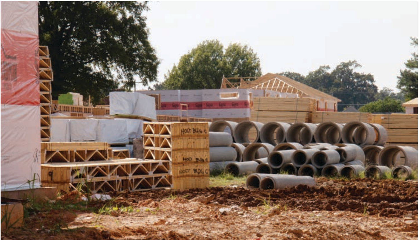
In addition to the influx of townhomes and condos in downtown and along the riverfront, affordable multi-family housing is under construction in North Little Rock's midtown as well.
