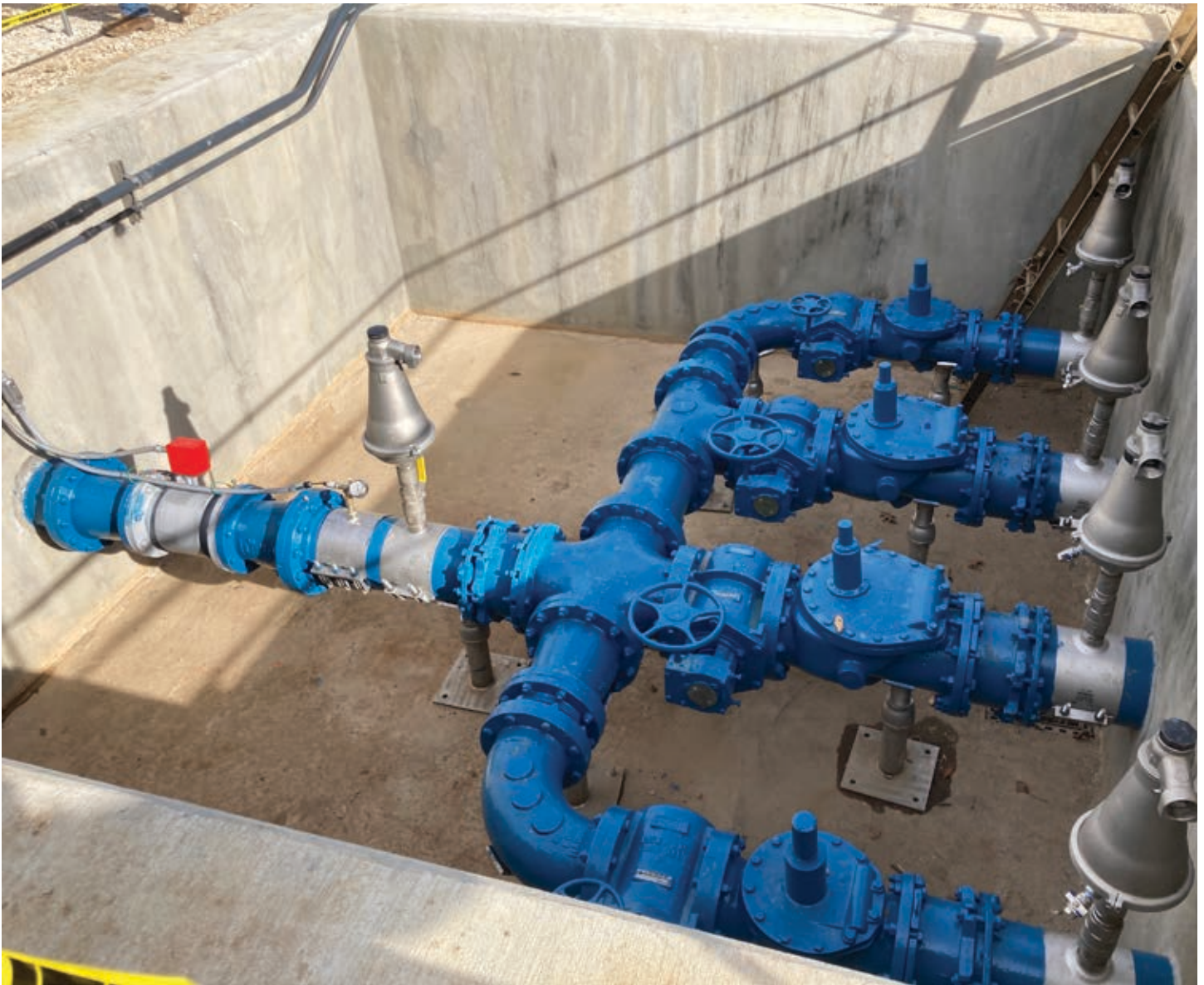
A completed pipe and valve gallery at West Fork's sanitary sewer lift station.
