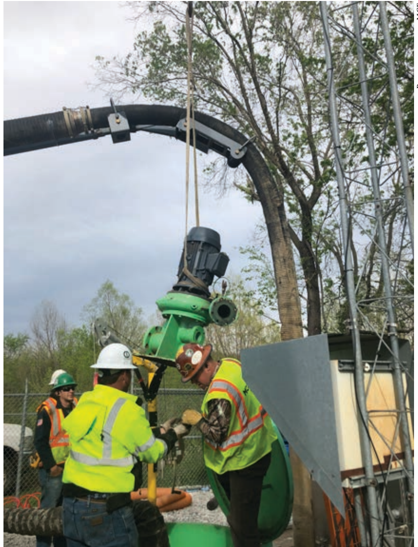
Workers install a new pump assembly at the city of Greenland's lift station.
