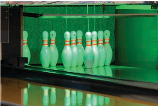
The city replaced the old mechanical “free fall” system with a string pin system, which is a big maintenance money saver.
